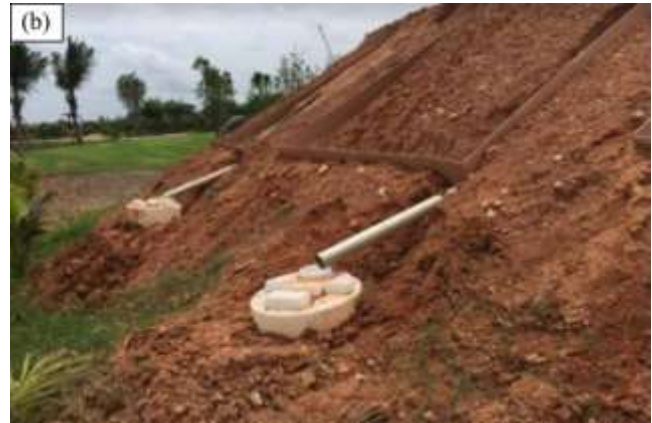
Embankment with soil and water run-off collection drums
